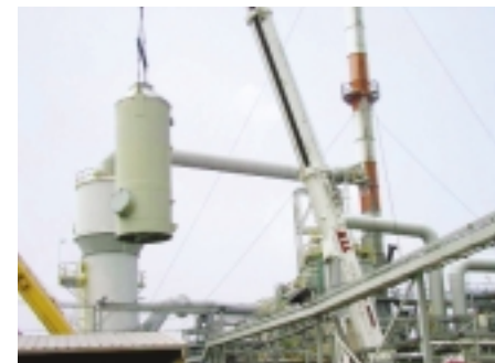
The finished product is placed into position at the Wurtland, Ky. facility with the assistance of Koch Knight's subcontractor ENERFAB Inc. of Cincinnati.
