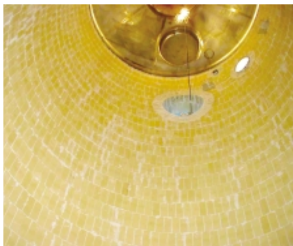
Because of the reduced tower size, Koch Knight was able to utilize a novel approach to construction on the DuPont job and line the tower in-house at the company's Canton, Ohio facilities.
