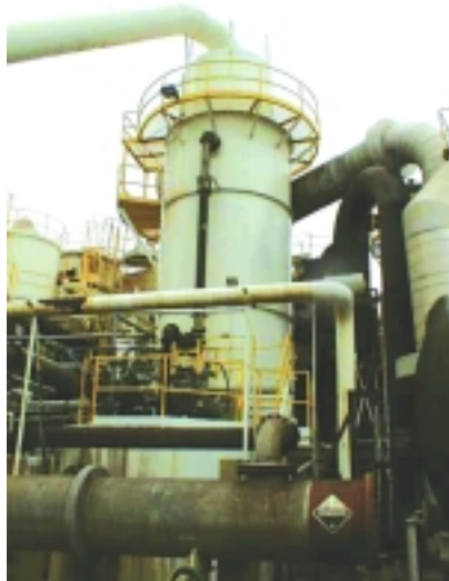
In 2000, a complete final absorbing tower was installed by the Knight Division of Koch-Glitsch at Marsulex's Oregon facility.
